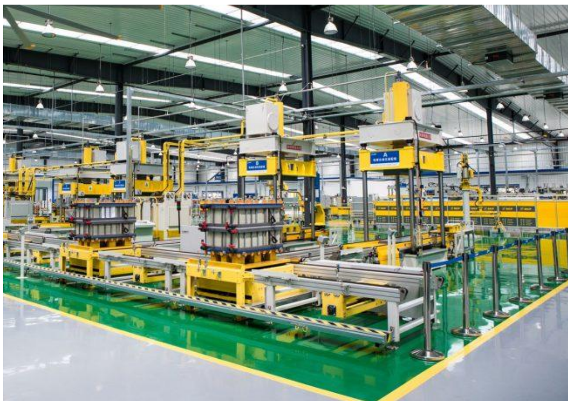
Vanadium redox flow battery storage
